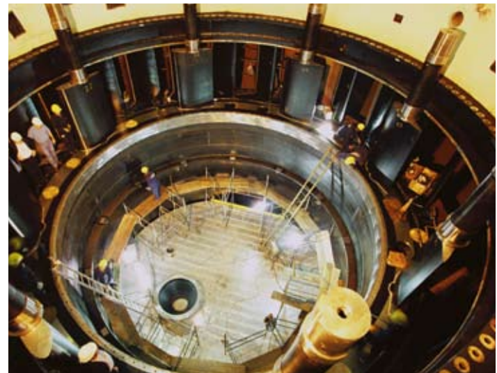
The rotor is one of the generator unity compounds and weighs 1,760 tons.
