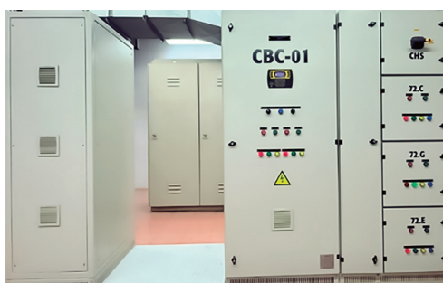
Novos painéis CBC-01 e CBC-02
