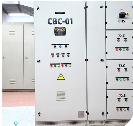
Novos painéis CBC-01 e CBC-02
